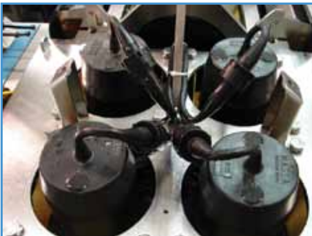
Transducers mounted inside of unit
